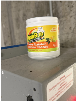
Odour absorber installed as a final support after odour neutralization.
