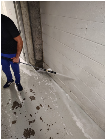
Directed rinsing of low walls and odour-retention zones.
